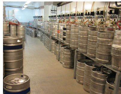
Walk-in Coolers and Freezers
