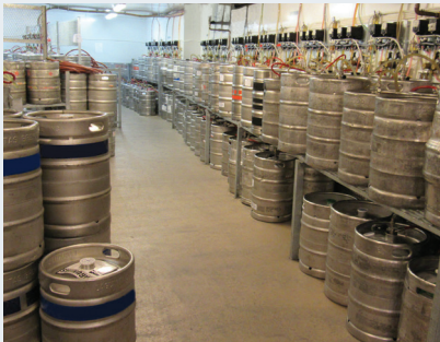
Walk-in Coolers and Freezers
