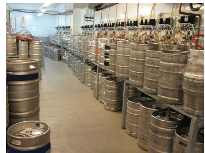
Walk-in Coolers and Freezers
