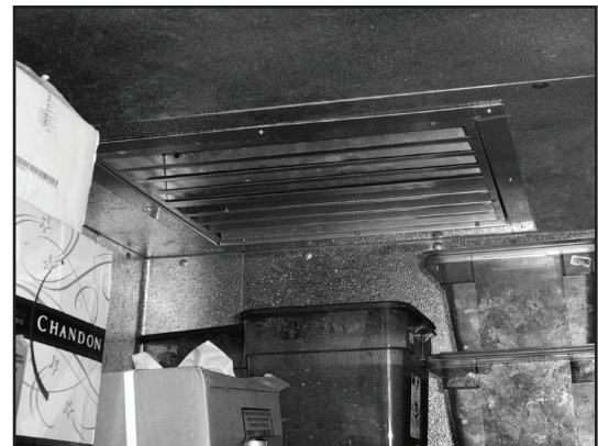
Inside view of an installed walk-in cooler.
