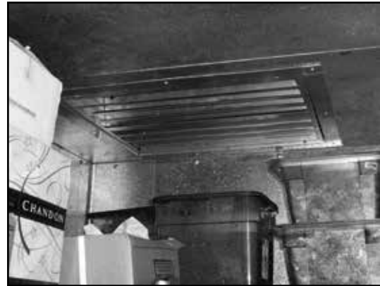
Inside view of an installed walk-in cooler
